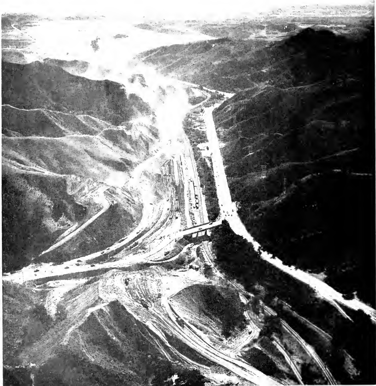
Looking southeasterly along grading operations for Golden State Freeway in Weldon Canyon. Son Fernando reservoirs skirted by Sepulveda Boulevard shown in background.
